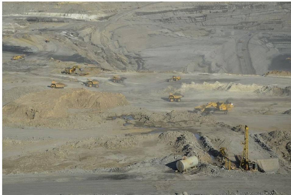
Figure 10. Drilling of dewatering well (lower right); the very permeable reefal debris can be seen as the white layer on the upper left part of the picture. (Source: GPPamintuan)
