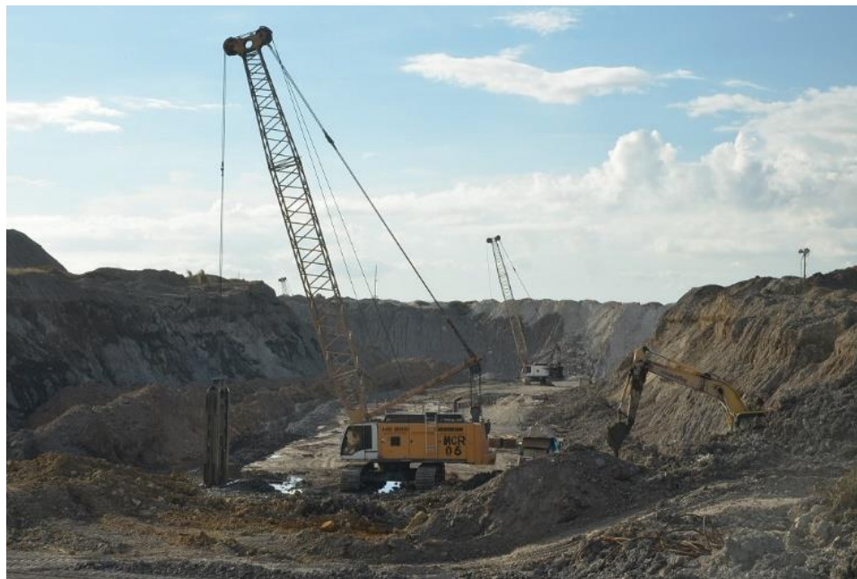
Figure 11. Installation of cut-off wall on the north side of the pit (Source: GPPamintuan)
